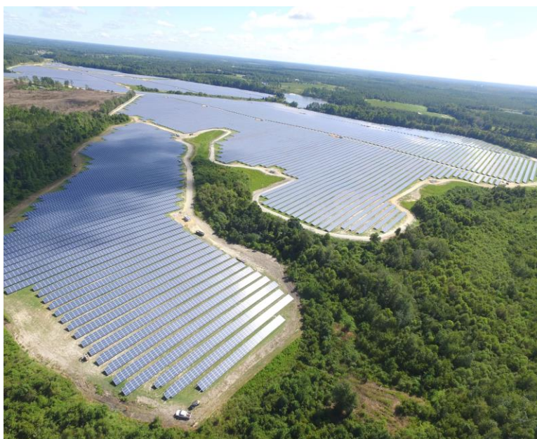
A ground-mounted solar system sited in a rural area.
